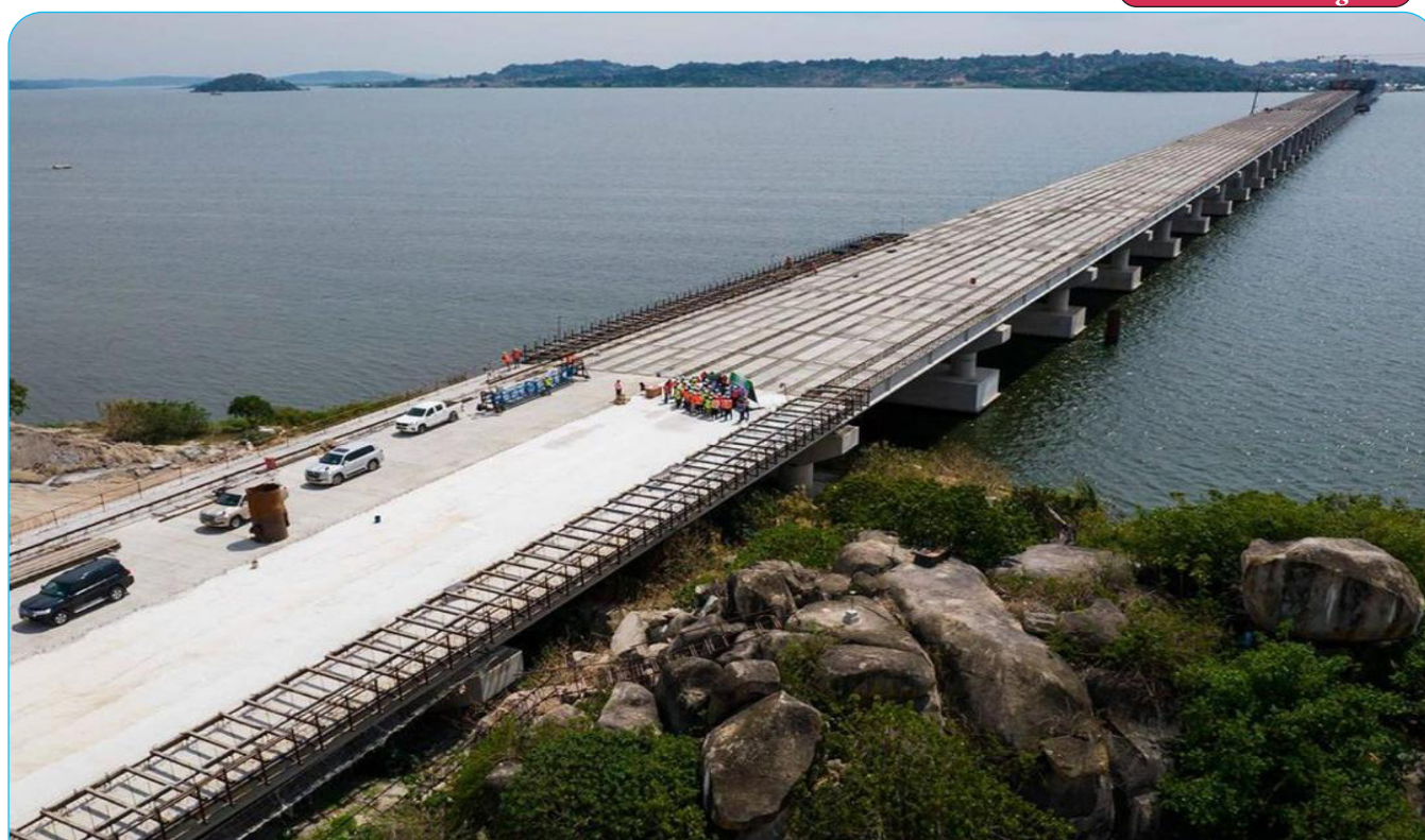
Kigongo - Busisi Bridge under construction in Mwanza Region (Photo: Ministry of Works)
